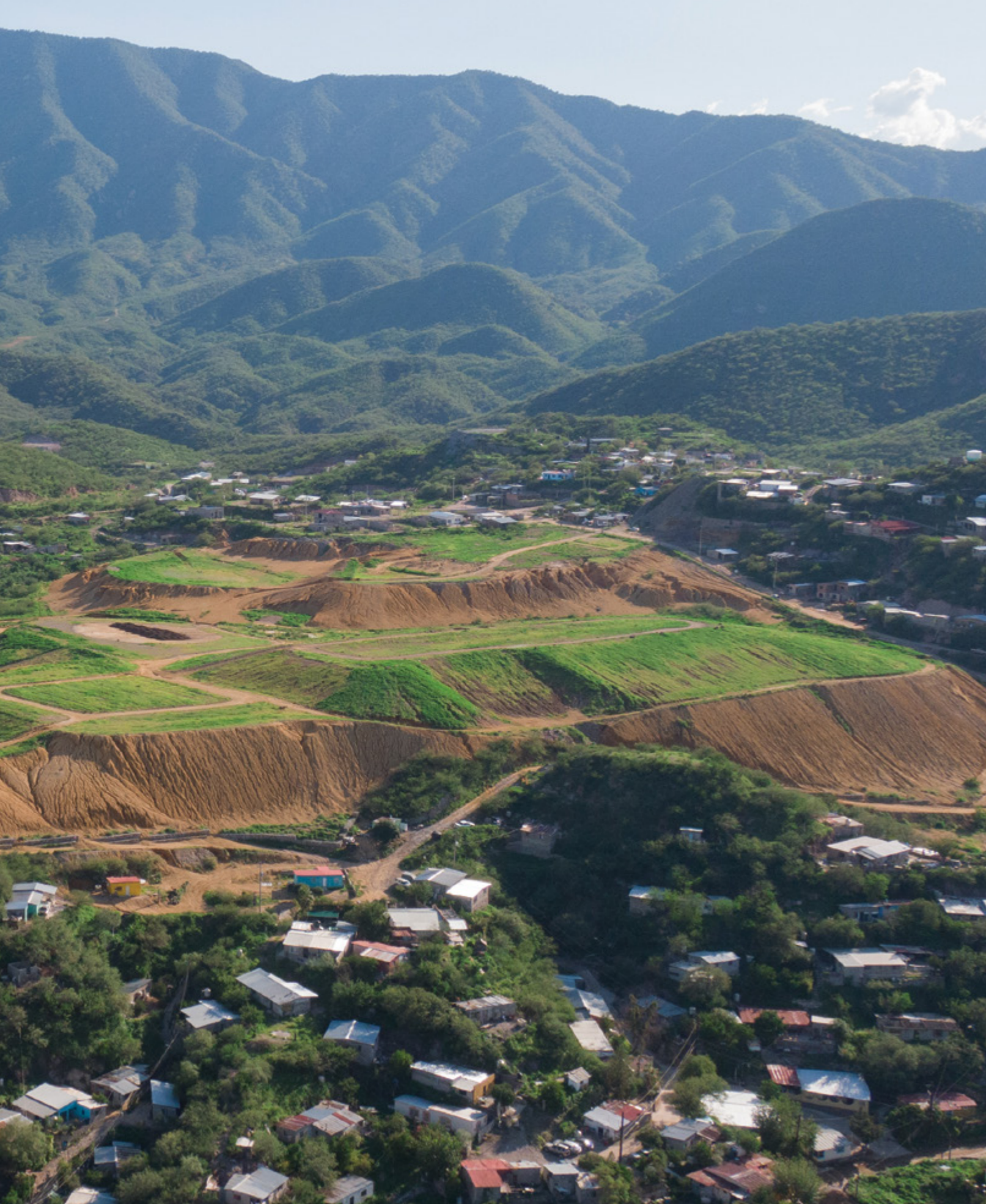
Remediation in progress of the old former Moctezuma Copper Company tailings deposit in Nacozari de Garcia, Sonora, Mexico.
