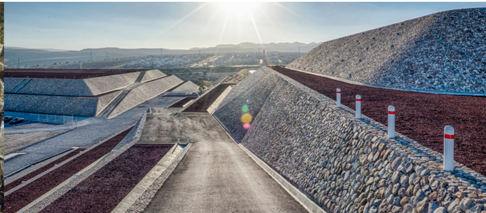
The soil remediation of the former plant in San Luis Potosí was carried out in accordance with the parameters set by the environmental authorities, and the Federal Commission for the Protection against Sanitary Risks (Cofepris) approved the containment plan, as per the regulations of the Ministry of Environment and Natural Resources (SEMARNAT).
