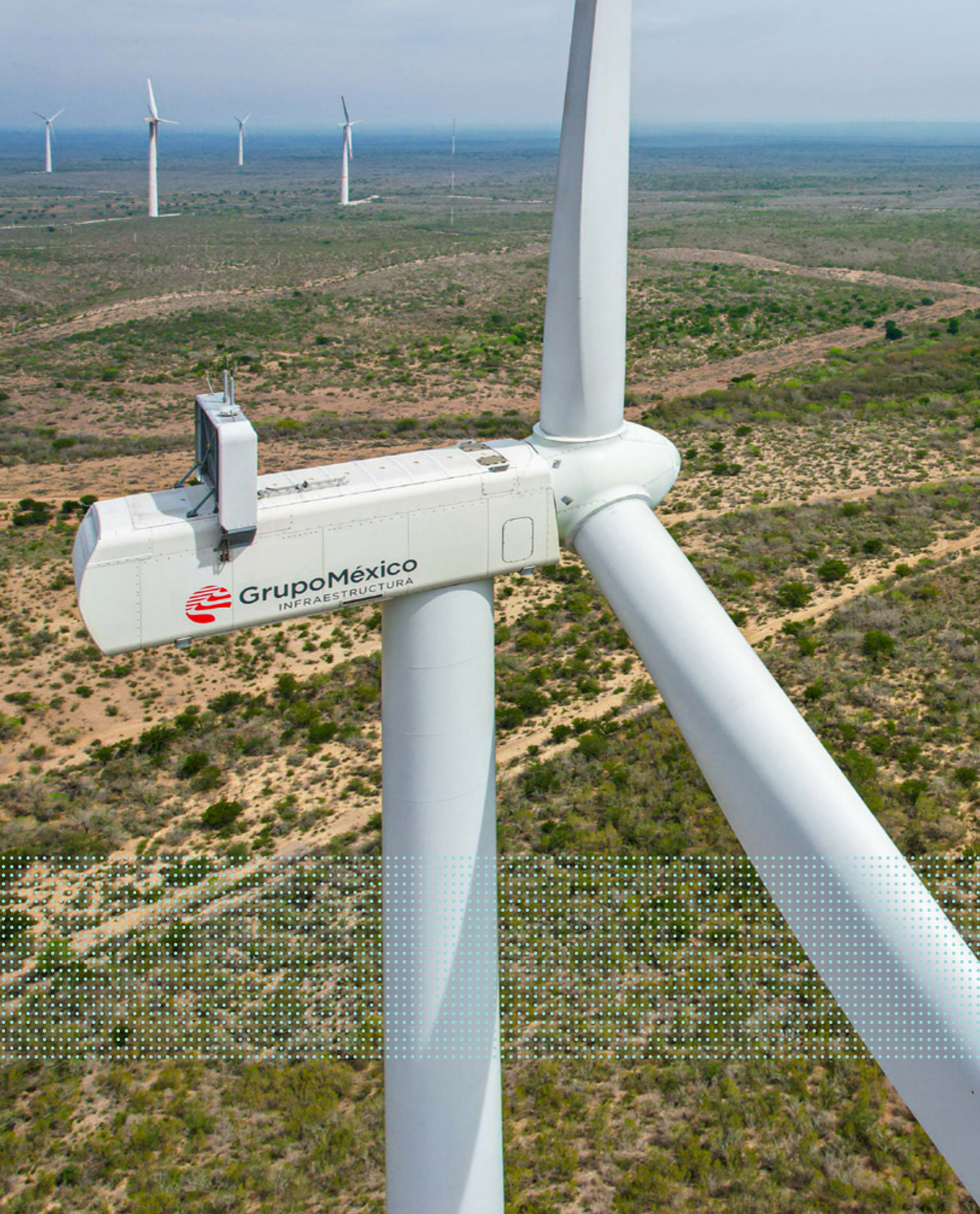
Fenicias Wind Farm with a production capacity of 168MW in Nuevo Leon, Mexico.
