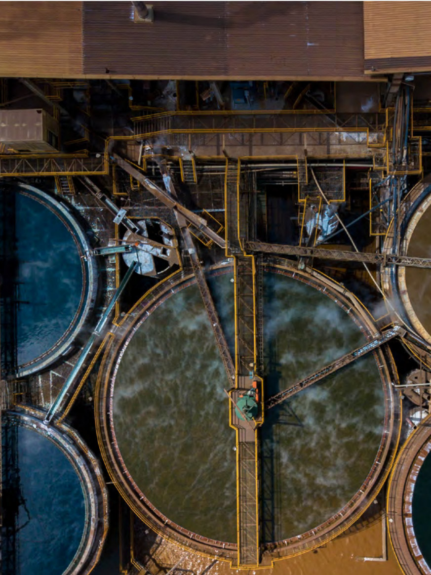
Thickener tanks of the Concentrator Plant, Cujajone Unit, Peru.
